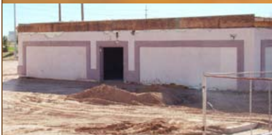
Below: IBC's modular buildings have been installed and need to be remodeled (electrical, roof, exterior, plumbing). $300,000 has been given; an additional $450,000 is needed to finish the buildings.
